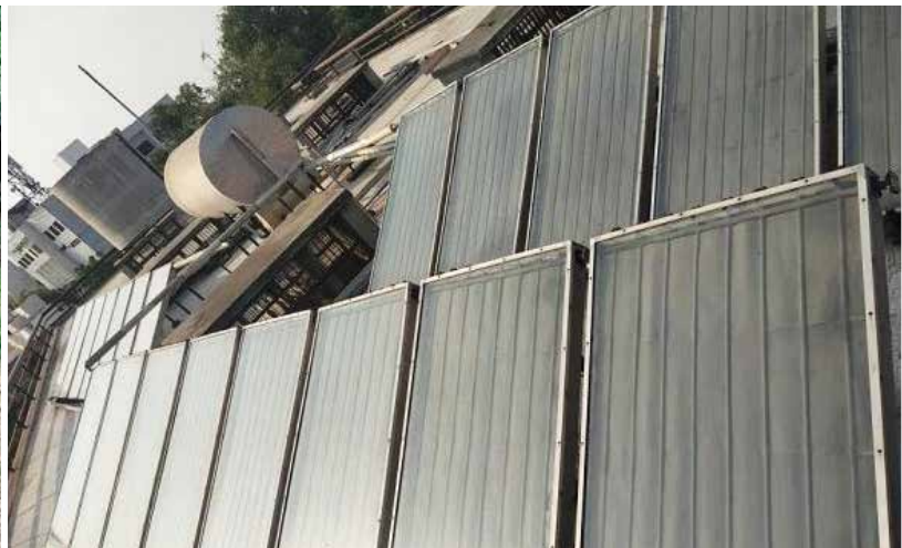
Example of Solar Heater Panel
